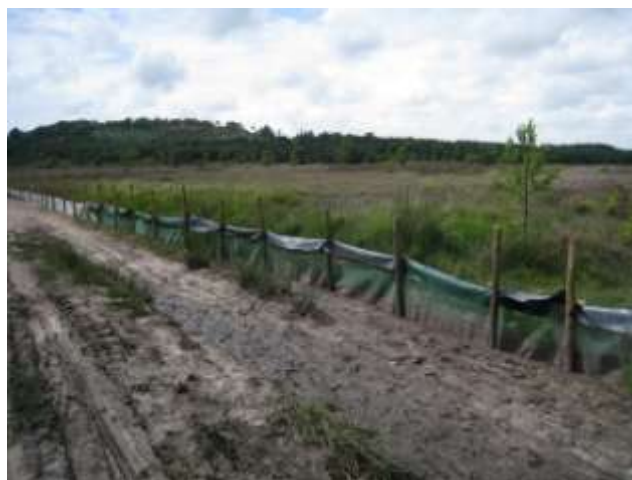
Fencing can prevent reptiles entering areas subject to earthworks or heavy plant movements
